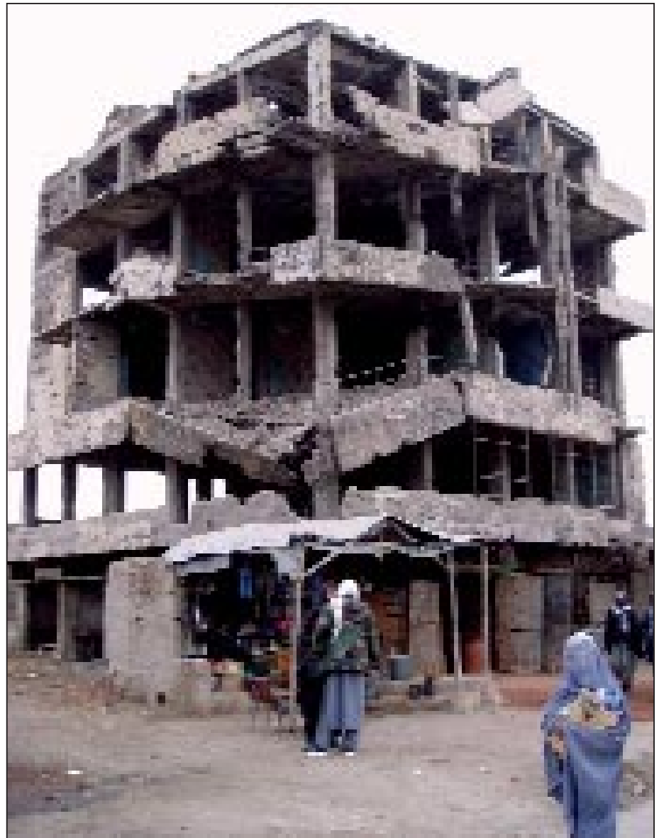
A typical structure within Kabul—virtually destroyed from warfare, but still being used.
